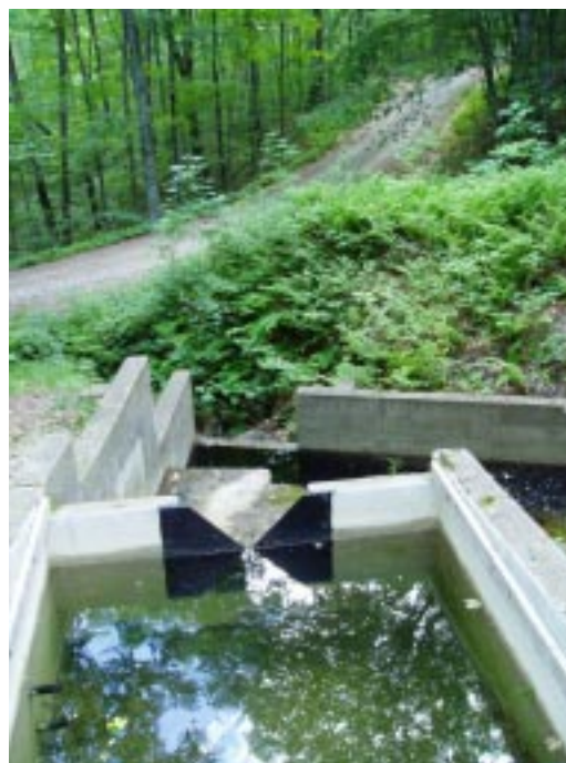
Concrete structures called "weirs" are used to measure water outflow from experimental watersheds. Stream height measurements, taken at the v-notch, accurately determine streamflow volume even when flow levels are very low.
